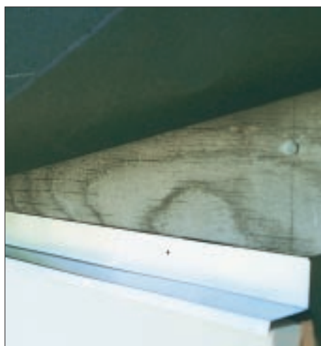
Figure 4. To prevent leaks at window heads, lap felt paper or housewrap over the cap flashing.
