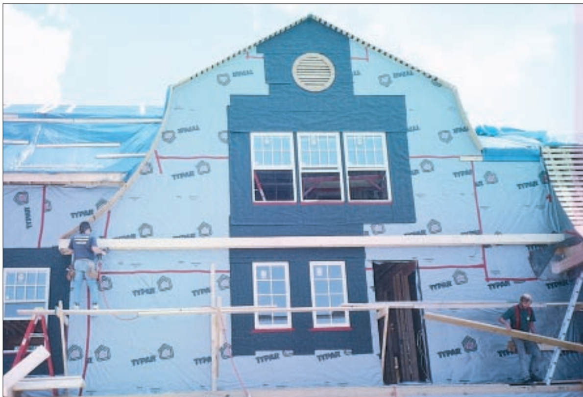
To protect this oceanfront home from wind-driven rain and surf spray, the builder has covered the housewrap around doors and windows with a self-adhering bituminous membrane.
