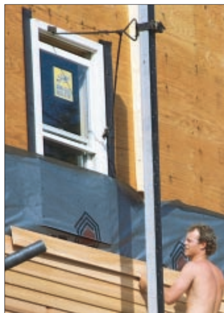
Figure 5. Because this carpenter has stretched the housewrap over the splines at the bottom of the window, wind-driven rain will be able to run down behind the housewrap onto the sheathing.
