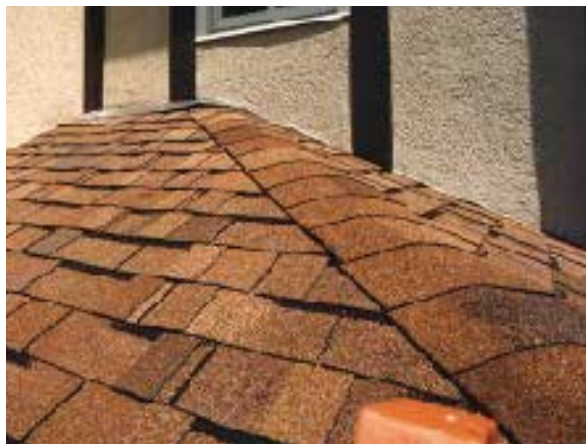
Figure 6. Contrary to the manufacturer's recommendation and common sense, the EIFS applicator butted the edge of the polystyrene directly against the roofing, with no caulk space or counterflashing.
